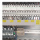
SCHNEIDER electricity parts
