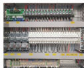
SCHNEIDER electricity parts
